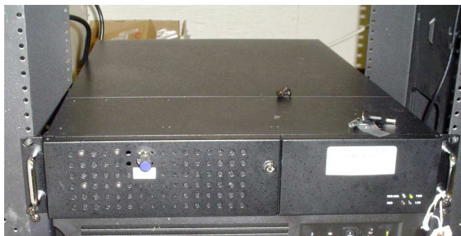
Figure 5. Inside rack-mounted METHUB Meteorological Data Receiver.
